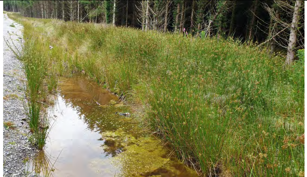
Pre-Existing Roadside Ponding and Poor Drainage Near the Forestry at T05
