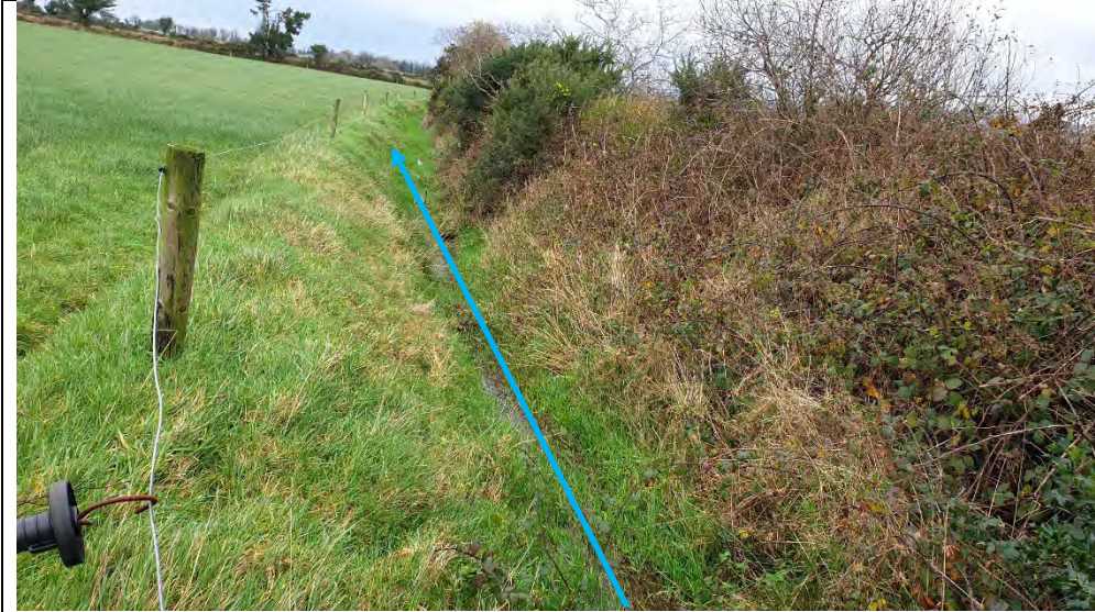
Existing Artificial Drainage Channel at Field Boundary near Central Area of the Site
