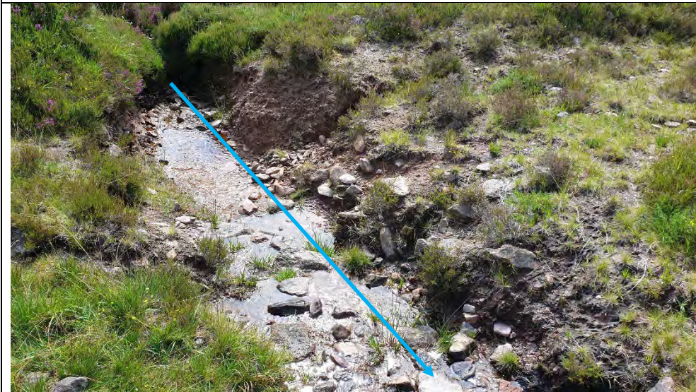
Natural Drainage Channel at the Western Commonage Area with Evidence of Erosion Visible
