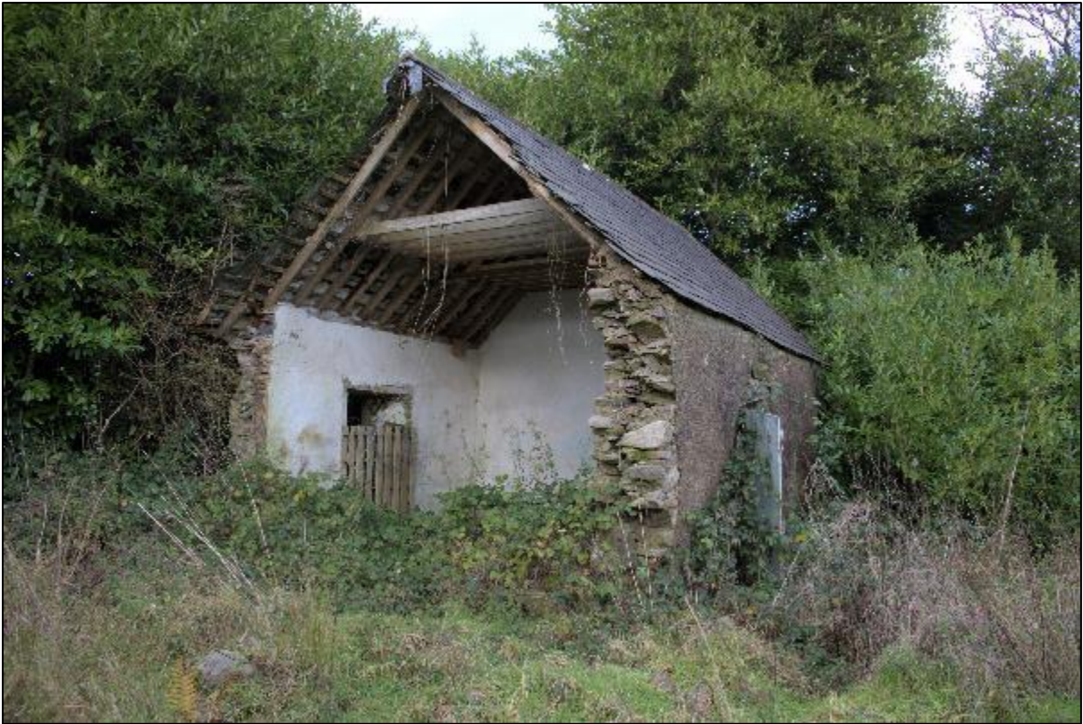
Plate 13.13: View of derelict farm building E in area to east of Turbine 9
